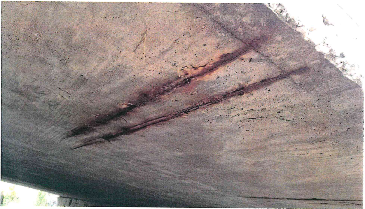
Exposed rebar in this photo shows that reinforcing steel was not properly resting on rebar chairs- poor construction practice
