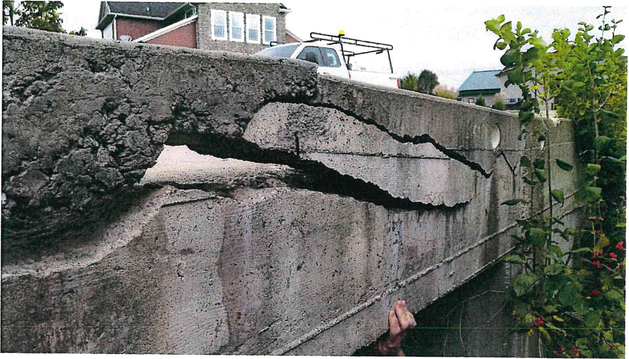
Evidence of structure under stress. Also note cold joint in curb – not a good construction practice.
